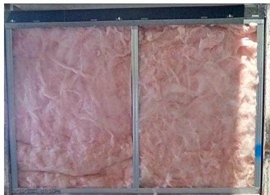
Figure 1: 3-inch leg ceiling runner (18-GA) and nom. 3-1/2 inch steel stud framing (25-GA, 24 inch OC) used to construct the wall. R13 fiberglass insulation fills the wall cavity.
